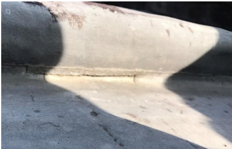
Photo 7 This photograph shows a typical in line crack in the cover-roll indicating the weakness of the lead along the fold line, and that it is fixed from movement by the roll
