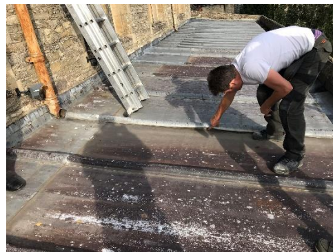
Photos 8 and 9 Typical illustration of a lead roll that looks in good condition. However after lifting it up, there is a crack about mid way along the lead sheet.
