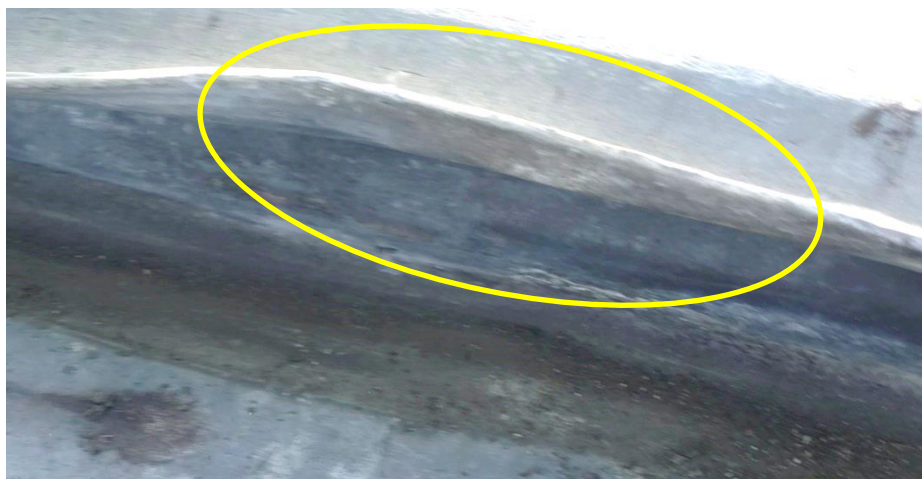
Photo 3 This photograph shows typical problems of in-line cracking in the lower rolls of the lead, beneath the cover-rolls
