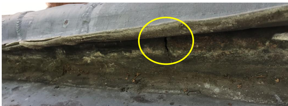
Photo 4 A further photograph showing transverse cracking in the lower lead roll.
